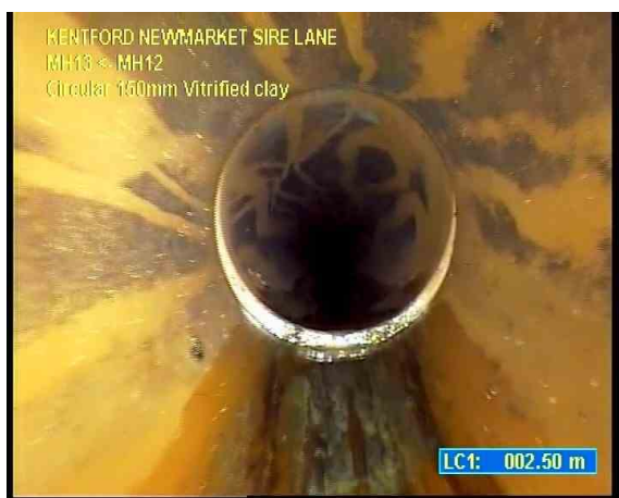
1, 00:00:25, 2.90 m Joint displaced, medium
