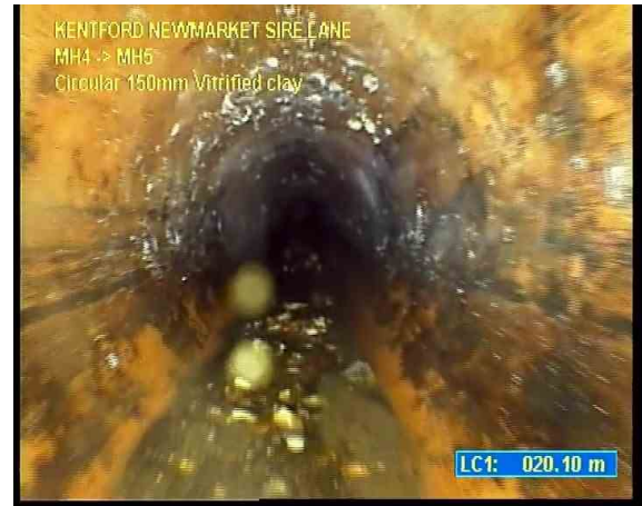
2, 00:04:12, 20.10 m Settled deposits, coarse at joint, 5% cross-sectional area loss, start
