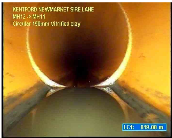
3, 00:02:33, 19.70 m Joint displaced, medium
