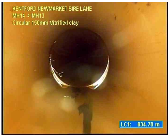
1, 00:05:38, 35.30 m Joint displaced, medium
