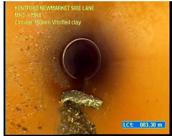
2, 00:00:46, 3.50 m Settled deposits, coarse, 5% cross-sectional area loss
