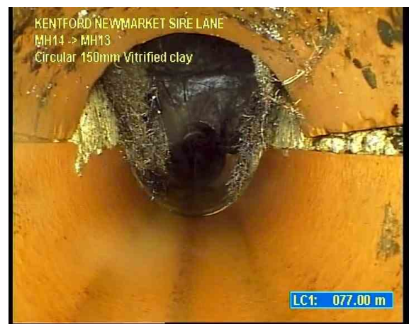
4, 00:22:26, 74.00 m Fracture, longitudinal at joint at 9 o'clock, start
