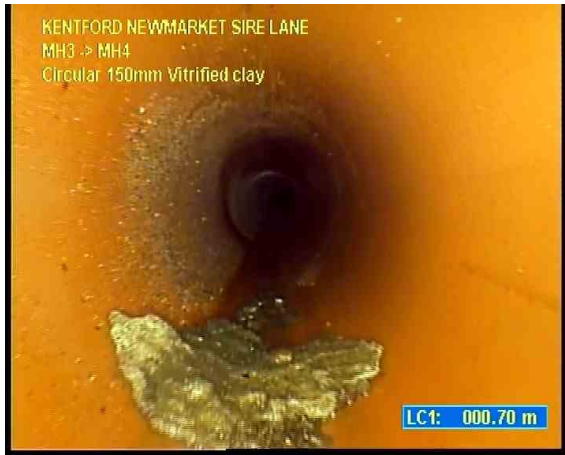
1, 00:00:18, 0.70 m Settled deposits, hard or compacted, 5% cross-sectional area loss
