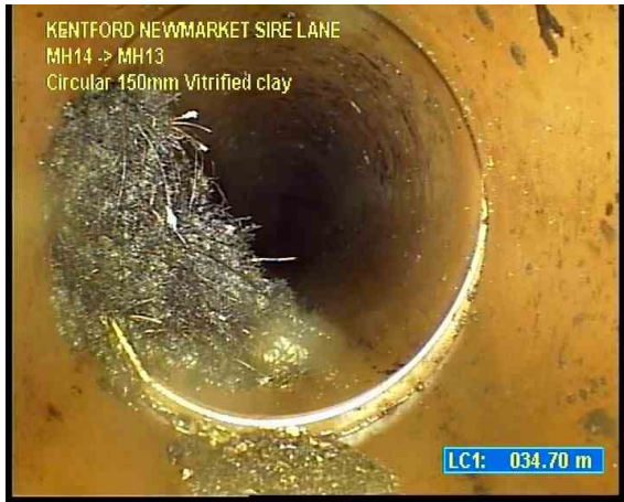
1, 00:07:01, 34.70 m Roots, mass at joint, 20% cross-sectional area loss
