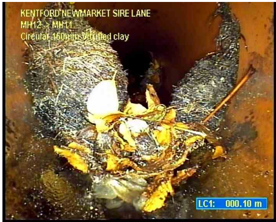
1, 00:00:25, 0.10 m Roots, mass at joint, 30% cross-sectional area loss, start
