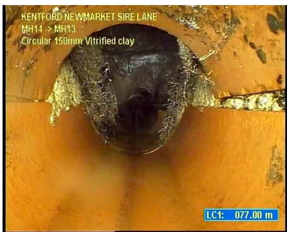
3, 00:22:26, 74.00 m Fracture, longitudinal at joint at 3 o'clock, start
