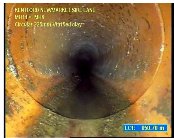
4, 00:22:02, 50.80 m Joint displaced, medium
