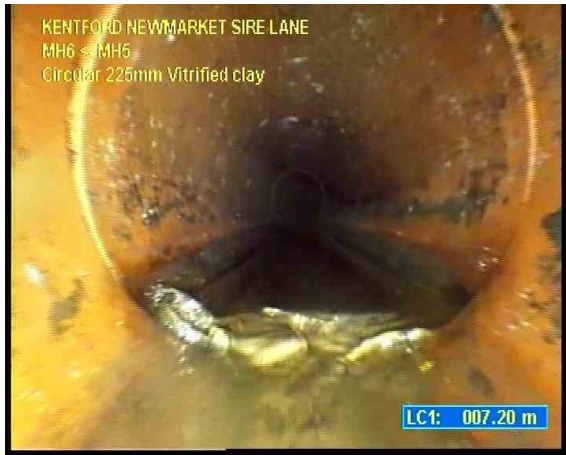
1, 00:01:04, 7.30 m Joint displaced, medium
