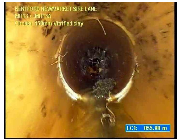
2, 00:14:30, 55.90 m Roots, mass at joint, 10% cross-sectional area loss, start
