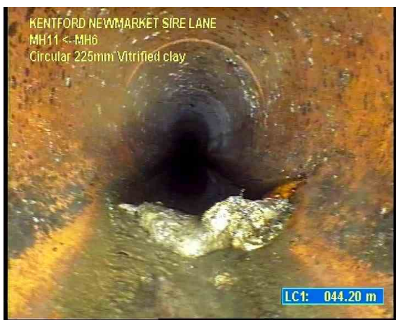
3, 00:16:41, 44.70 m Settled deposits, hard or compacted, 10% cross-sectional area loss
