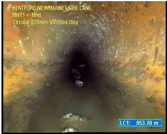
5, 00:25:34, 53.80 m Settled deposits, coarse at joint, 5% cross-sectional area loss, start
