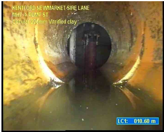
1, 00:01:29, 10.90 m Joint displaced, medium
