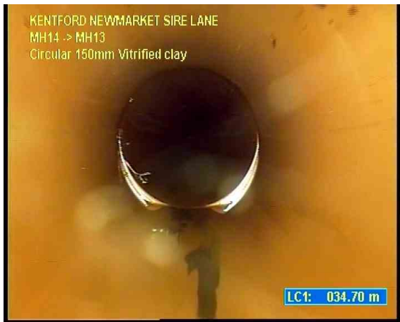
1, 00:05:38, 35.30 m Joint displaced, medium
