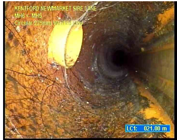
2, 00:03:03, 21.00 m Connection defective, connecting pipe is intruding at 12 o'clock, 150mm dia, intrusion: 10%
