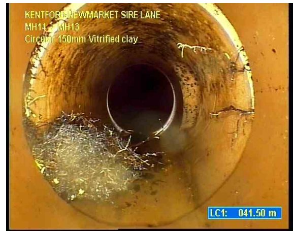
2, 00:06:42, 41.50 m Roots, mass at joint, 5% cross-sectional area loss
