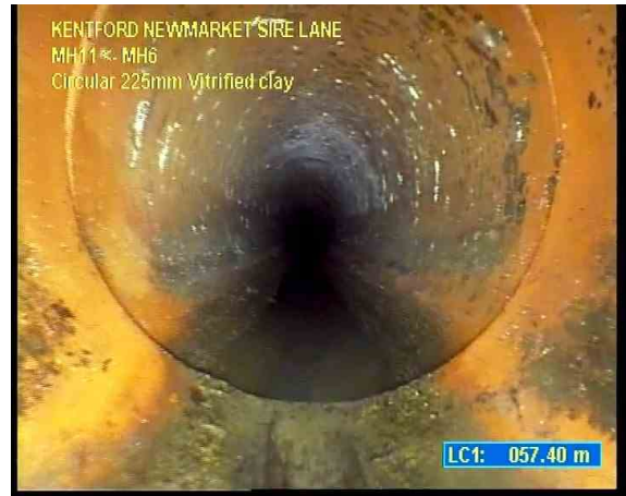
6, 00:26:07, 57.50 m Joint displaced, medium
