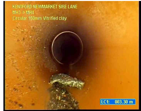
2, 00:00:46, 3.50 m Settled deposits, coarse, 5% cross-sectional area loss
