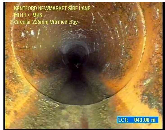
2, 00:14:56, 43.30 m Joint displaced, medium
