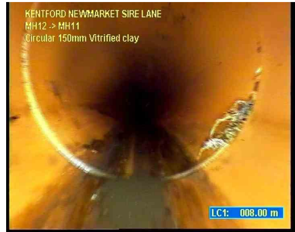
2, 00:01:29, 8.10 m Roots, fine at joint
