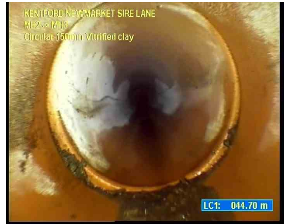
2, 00:07:38, 44.70 m Joint displaced, medium
