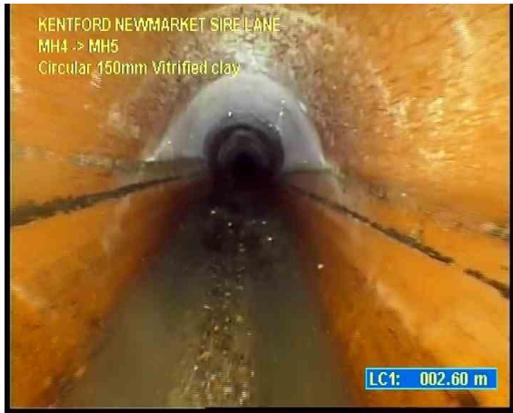
1, 00:00:35, 2.60 m Settled deposits, fine at joint, 5% cross-sectional area loss, start
