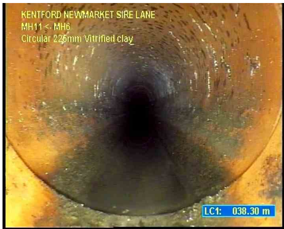
1, 00:10:13, 38.50 m Joint displaced, medium
