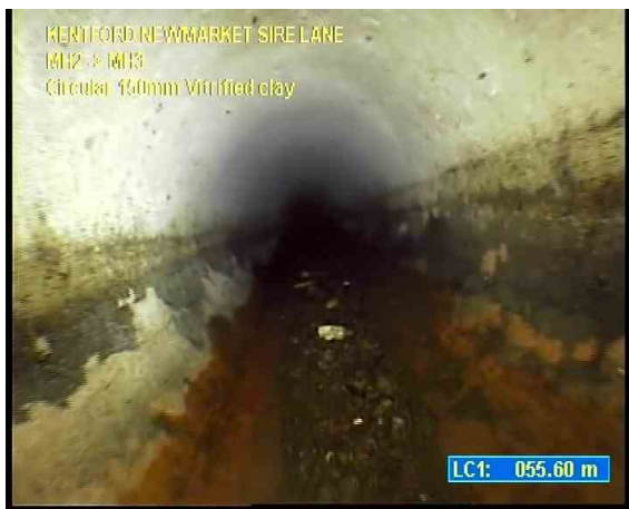
3, 00:09:29, 55.60 m Settled deposits, coarse at joint, 5% cross-sectional area loss, start
