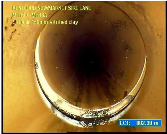
1, 00:00:27, 2.30 m Joint displaced, medium
